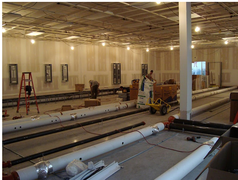
Figure 5. Cooling pipes being laid out below what will be the machine room floor during the construction of the data centre.
