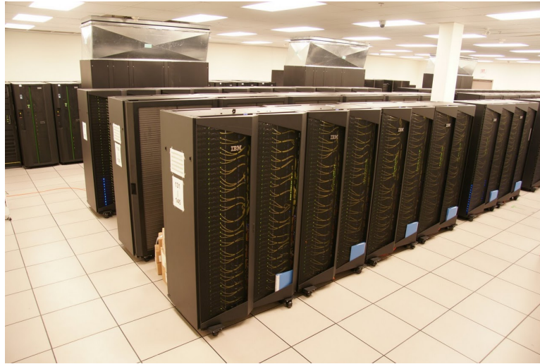
Figure 2. Partial view of the computer room in the SciNet data centre. In front, the GPC iDataPlex racks; at the very back, the TCS and disk.
