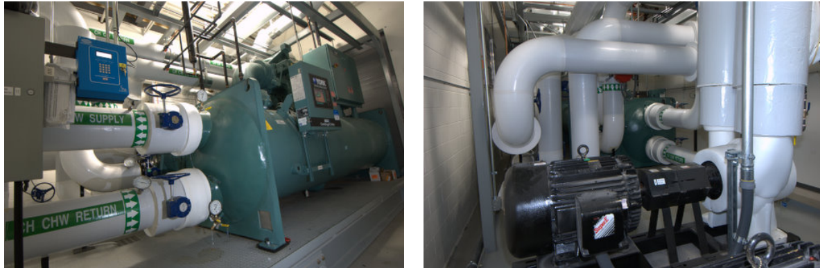
Figure 3. The 735T centrifugal chiller used in the SciNet datacentre, with some of the associated plumbing.
